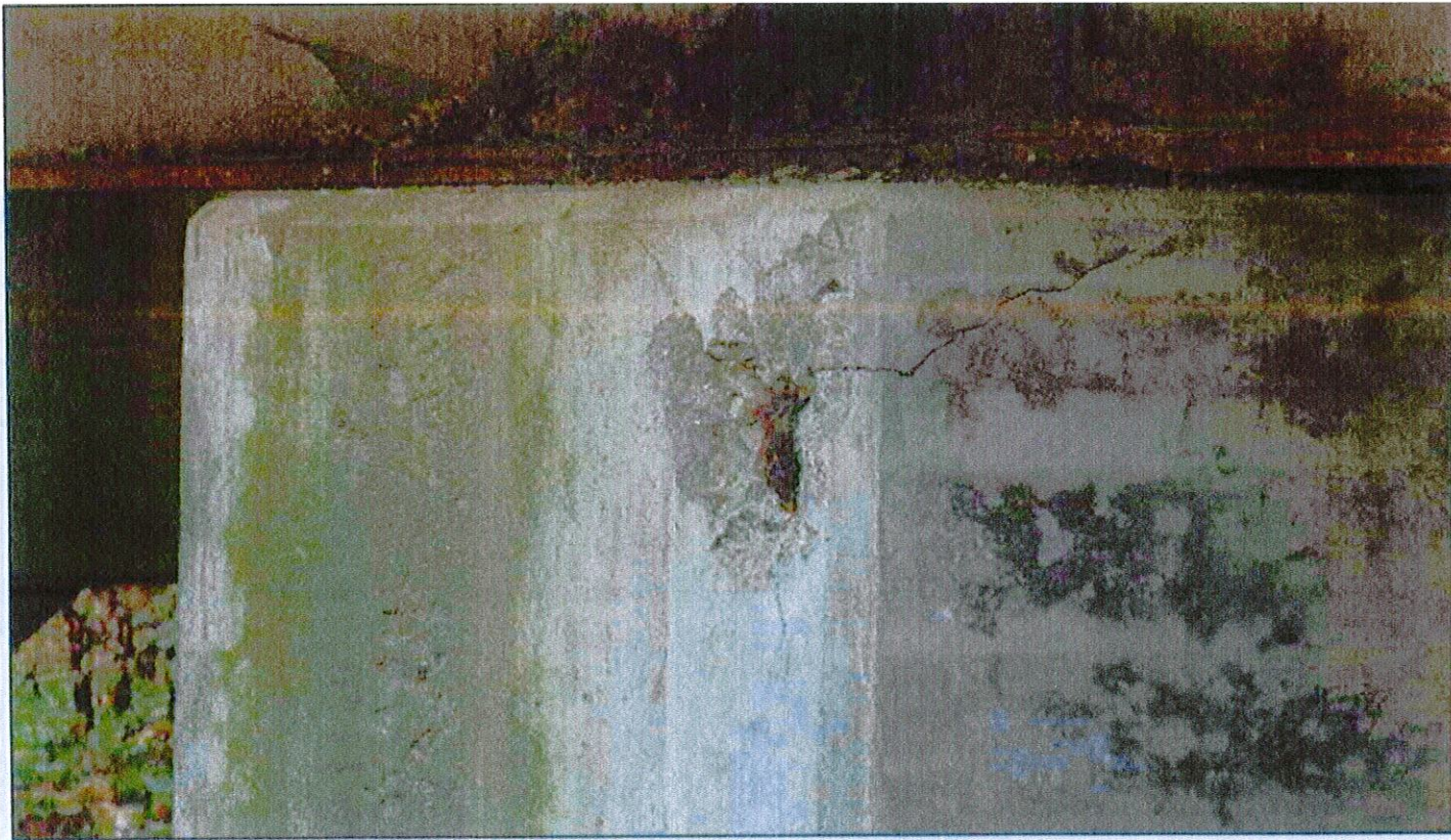
SPALL IN THE LEFT END OF PIER 1 CAP
