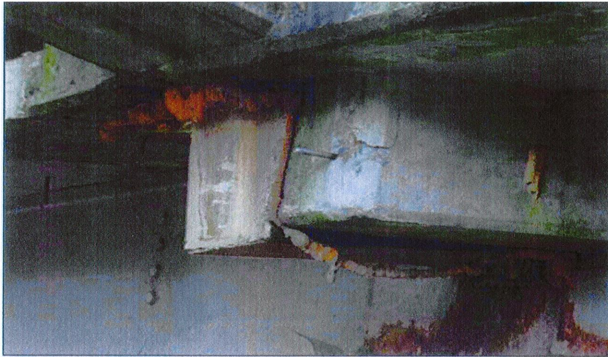
SPALL IN SPAN 2 DECK OVERHANG, LEFT SIDE AT PIER 1
